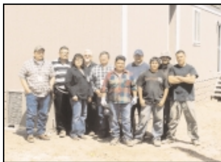
Work crew takes a break from the preparation of new housing units.
